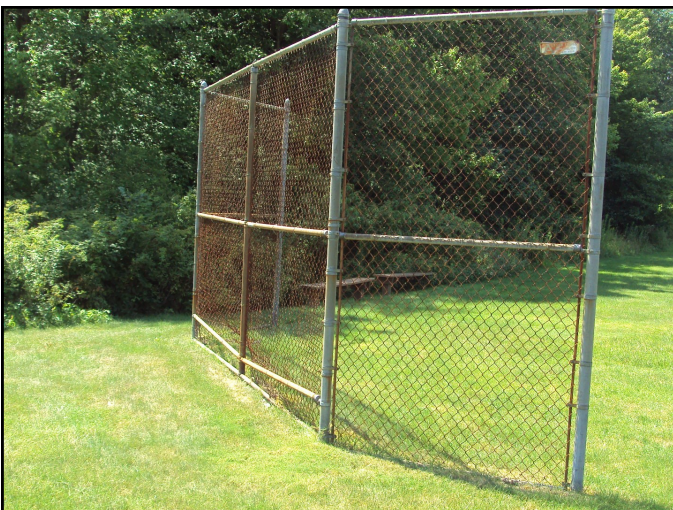
Rec Area / Backstop - (Repair recommended)
